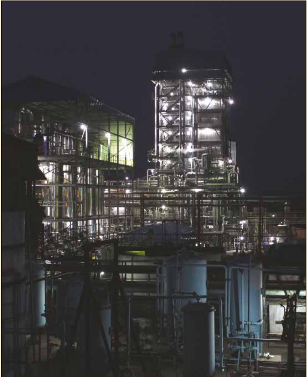
Incineration Boiler - Sameerwadi, Karnataka
